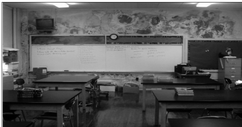
Figure 4. Water Damage and Black Mold, Johnson High School Classroom
